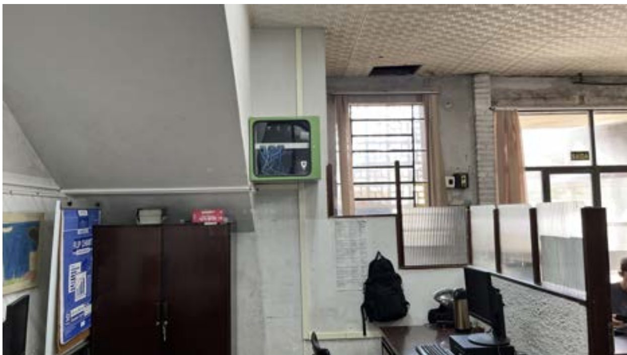
Figura 5 – Rack ( R ) e as canaletas nas paredes
